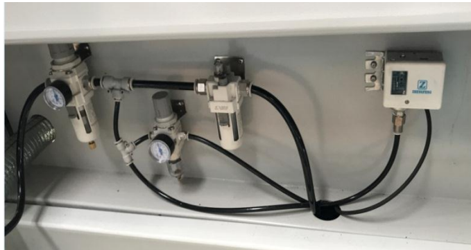
Instruments: 1.2. Air filter 3. Air pressure adjustable 4. Air pressure monitor
